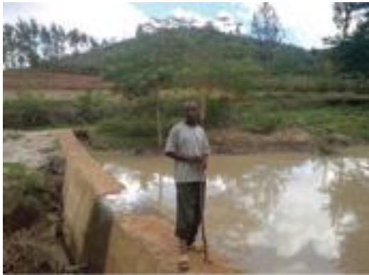
Water pans trap and store water
