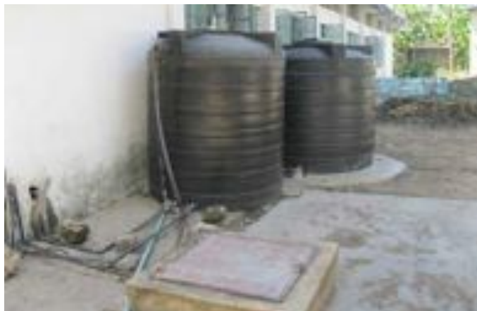
Tanks for water storage
